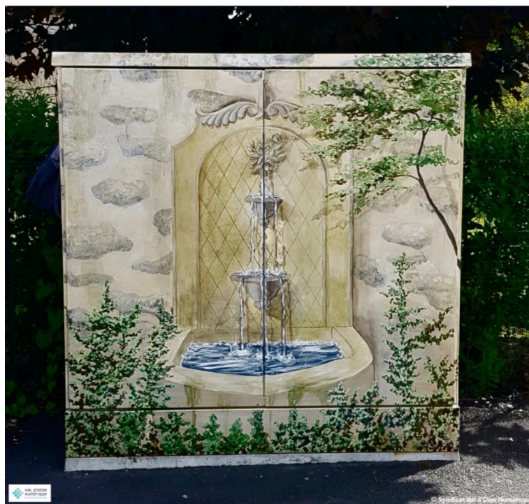
Example of a cabinet from Val d'Oise
